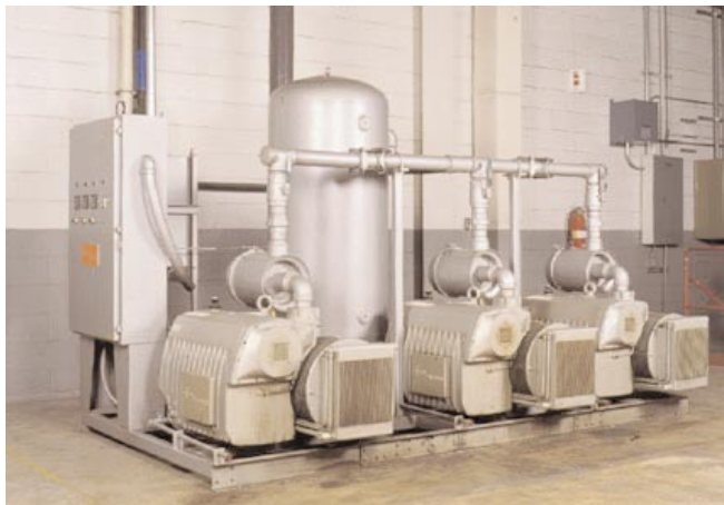
Central vacuum system site is mezzanine level above printing floor. Controller at left selects among 3 pumps to serve as lead, peak and backup unit, later alternates functions so pumps wear evenly. Centered behind pumps is large cylindrical reservoir.
